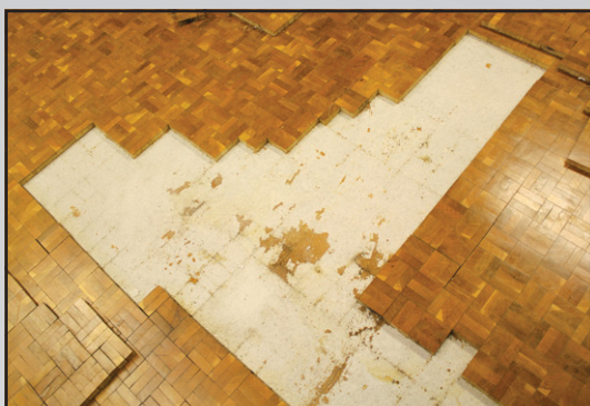
Pic. 7 Loose pieces of floor with old adhesive
